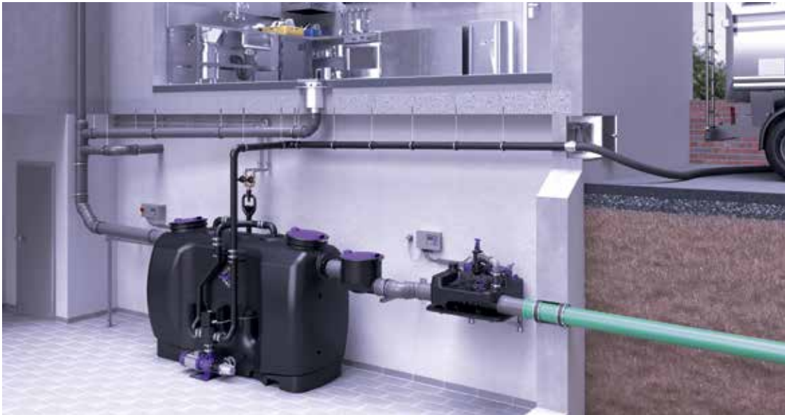
Ecolift L Bypass (SWA) in a commercial building below the backwater level after a grease separator
